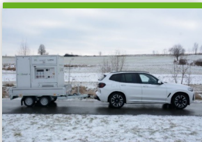
Mobile emergency power
