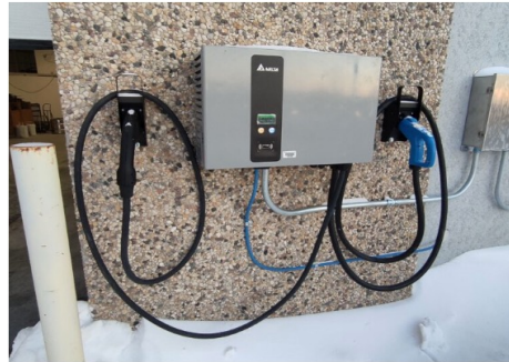
Repurposed battery DC fast charger
